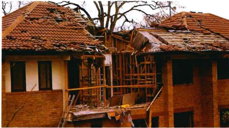
Mr Smith's home with its roof missing
